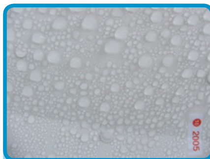
pict. 1A Condensation in the cabinet: on cabinet's surface
