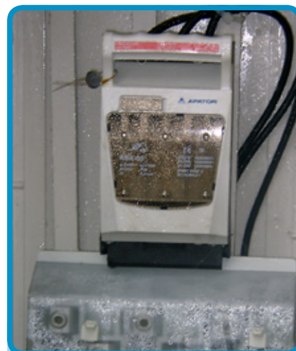
pict. 1B Condensation in the cabinet: on devices
