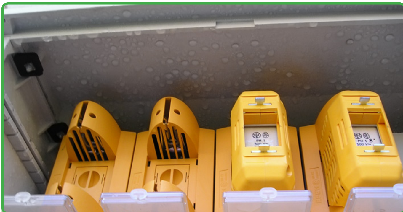
pict. 1 Water vapour condensation inside cabinet
